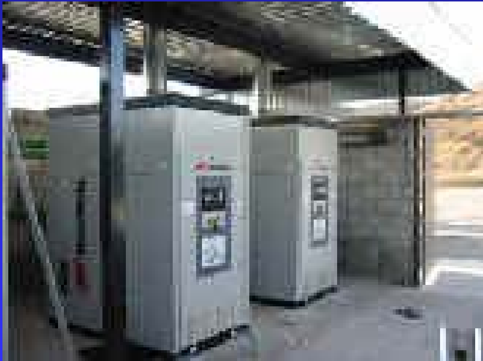
280 kW Microturbine Plant San Diego
