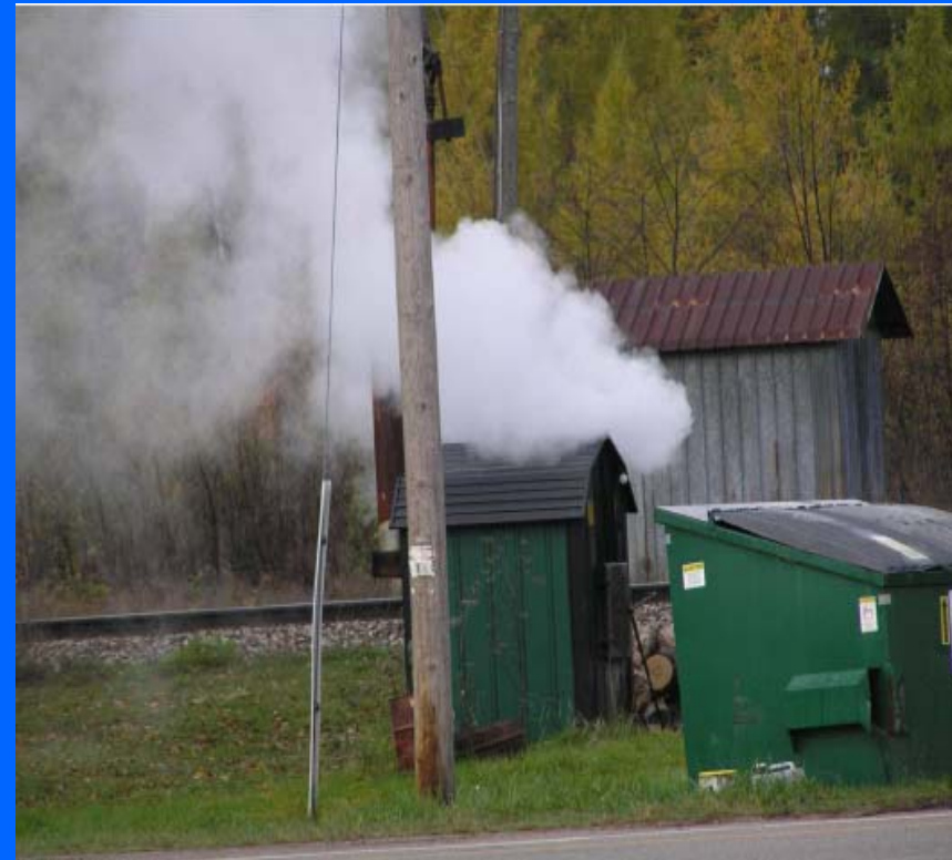
Outdoor wood boiler, Jericho, VT
